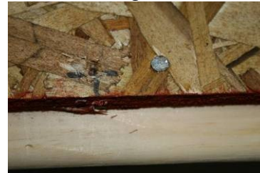
Photo 25: Relocated Nail at Damaged Edge
