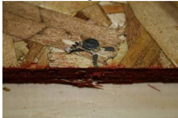
Photo 24: Edge Blow Out
