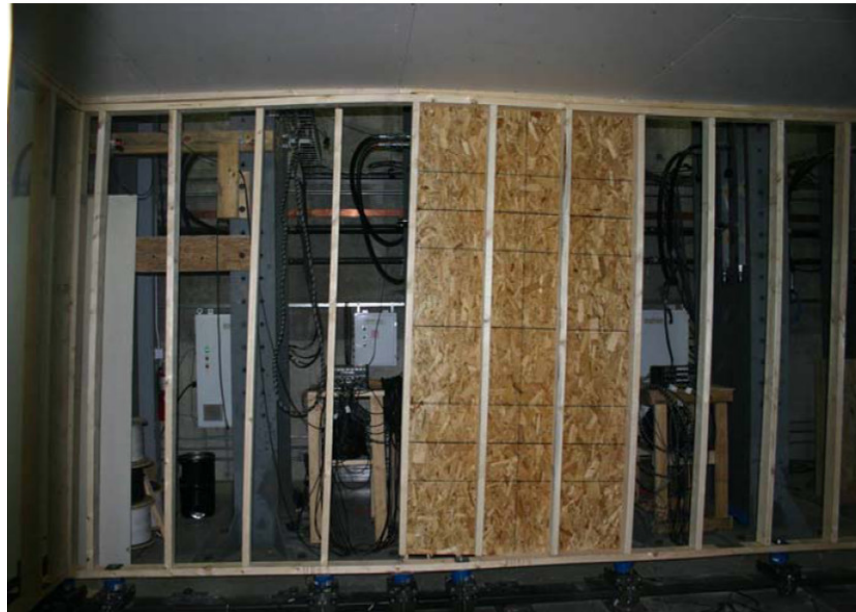
Figure 10: SBCA Research Institute Wall Failure (SBCARI T-IRC)
